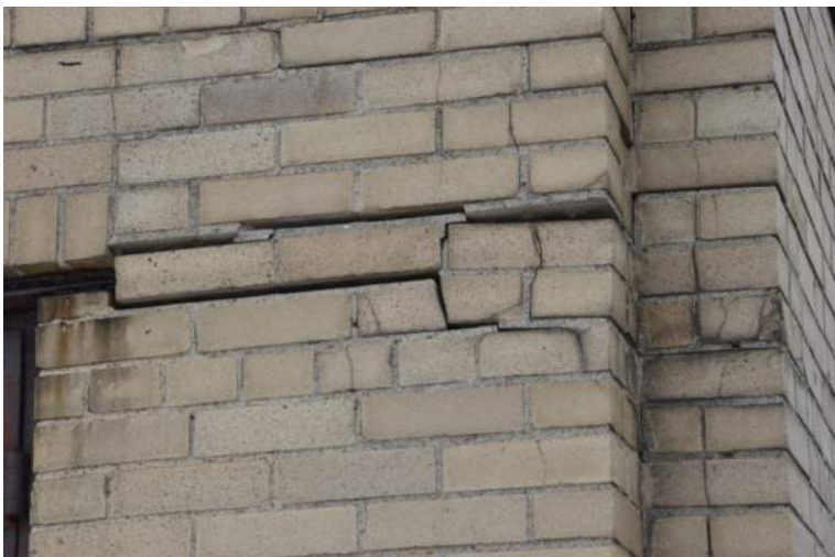
Photo 1-4c: Masonry Lintel with oxide jacking
