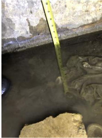
Photo 4-9: Service Chase Foundation Wall Standing Water
