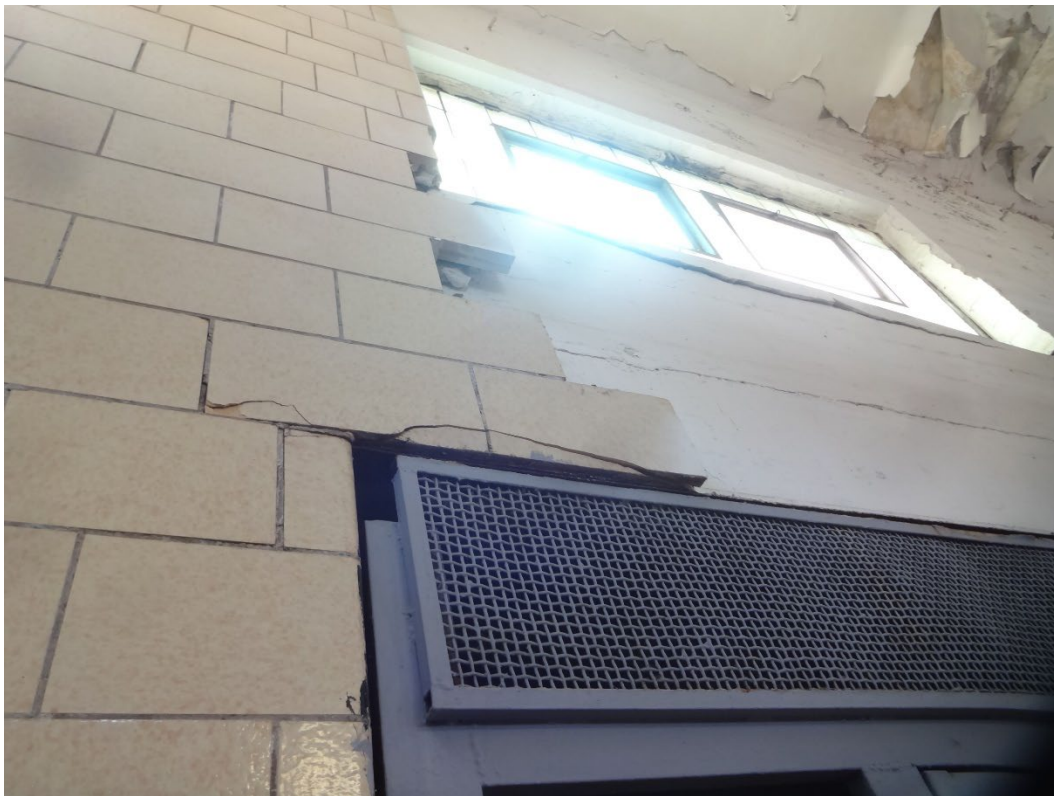
Damaged masonry adjacent to area of interior masonry previously removed.
