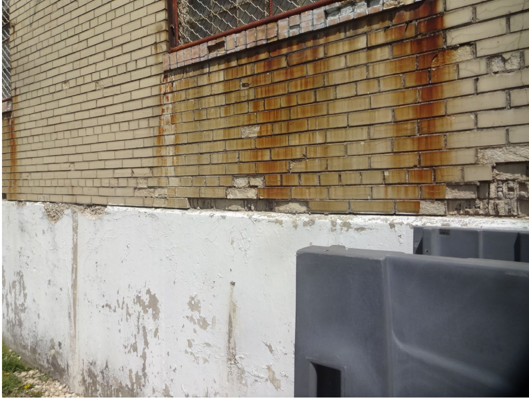
Typical location, damaged exterior masonry at grade level.
