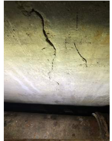
Photo 4-4b: Service Chase Foundation Wall Long Vertical Crack
