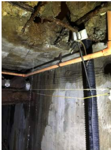
Photo 4-6: Service Chase Foundation Wall Horizontal Crack
