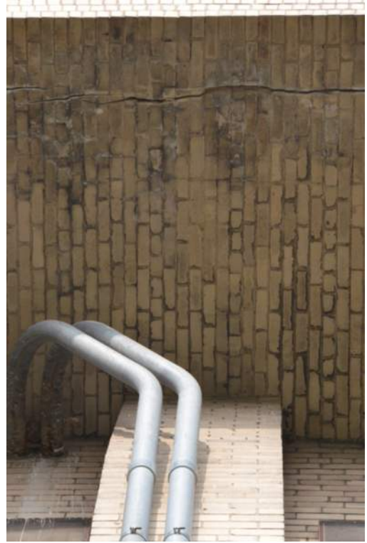
Photo 1-3c: Masonry South Arch crack
