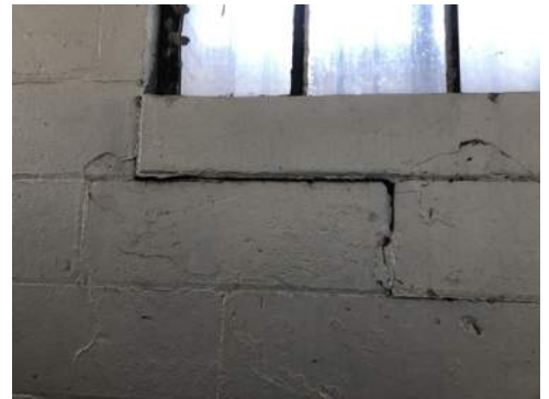
Photo 2-25: Interior Guard Rm North exterior wall crack
