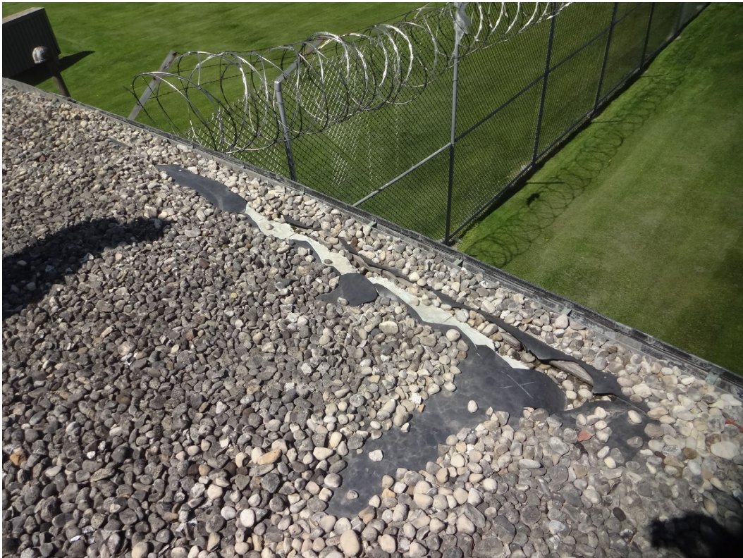
Typical location, damaged roofing at building edge.
