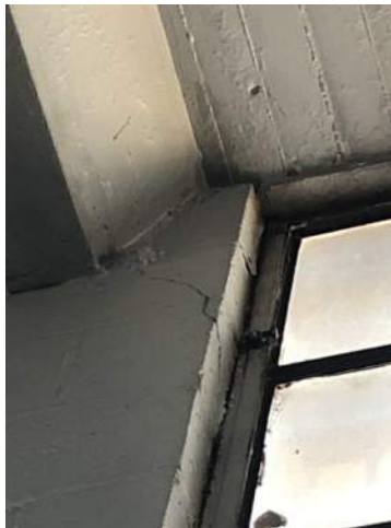
Photo 2-24: Interior Guard Rm Beam North exterior wall crack
