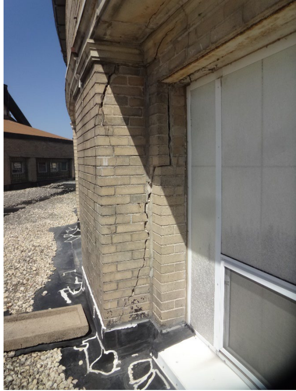
Typical location, cracked masonry.
