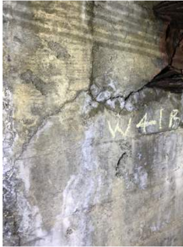
Photo 4-2: Service Chase Foundation Wall Horizontal to Vertical Crack
