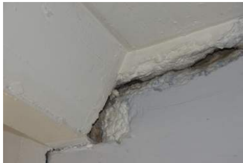
Photo 2-4: Interior B House East Beam to North Wall from Cell Wall cracks
