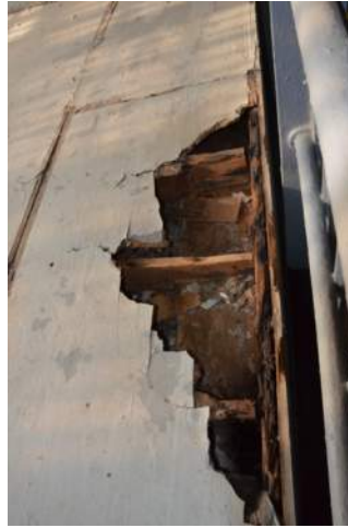
Photo 2-19: Interior C House Shower Roof Deteriorated
