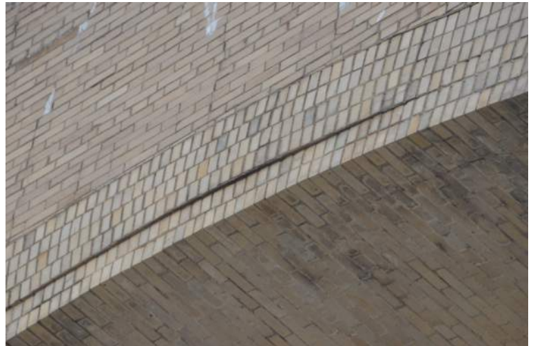
Photo 1-3i: Masonry North Arch brick separation
