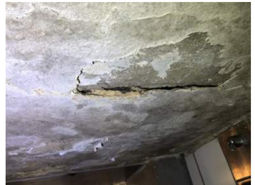
Photo 2-17: Interior B House shower ceiling
