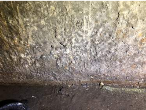
Photo 4-8: Service Chase Foundation Wall Spalling & Saturation
