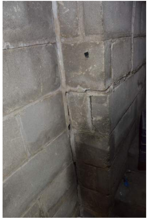
Photo 1-3e: Masonry South Arch Interior wall crack east side
