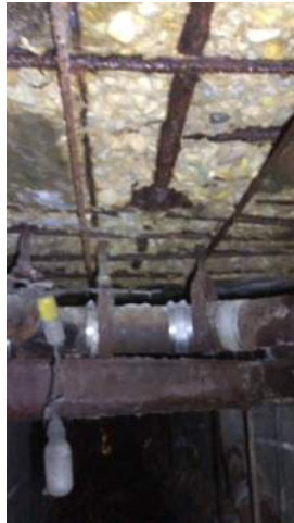
Photo 4-12: Service Chase Ceiling Slab Completely Exposed Rebar no Cover
