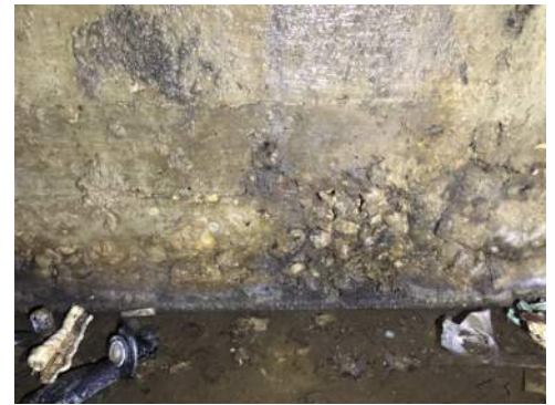
Photo 4-7: Service Chase Foundation Wall Honeycomb & Saturation
