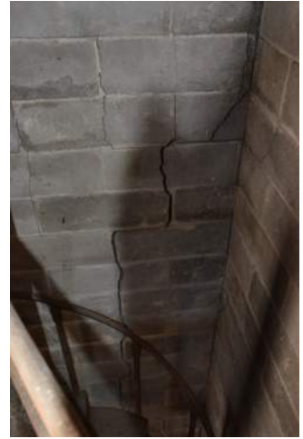
Photo 2-37: Interior South West Stairwell vertical wall crack
