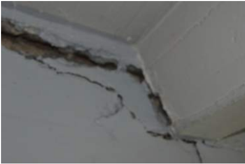
Photo 2-12: Interior E House West Beam to North Wall from Cell Wall cracks
