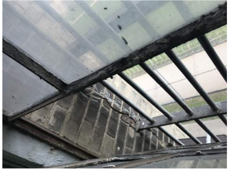
Photo 1-5f East Wall Window Condition
