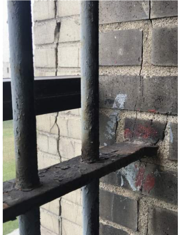
Photo 1-5b: Masonry Fine vertical cracks at Barred Grille
