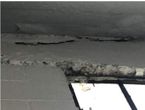
Photo 2-23: Interior Guard Rm cracks on exterior wall requires further investigation.
