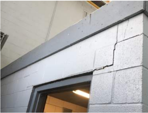
Photo 2-18: Interior C House Shower Entry wall cracks
