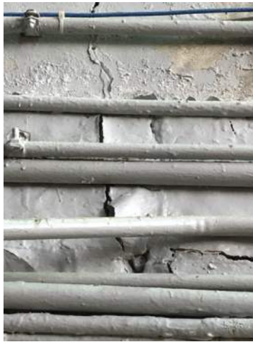
Photo 2-1b: Interior B House North Wall vertical crack detail
