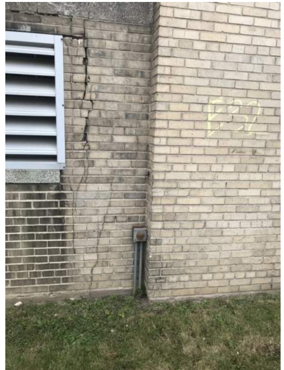
Photo 1-4b: Masonry Lintel with oxide jacking
