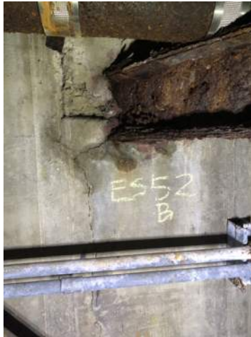
Photo 4-4a: Service Chase Foundation Wall Long Vertical Crack
