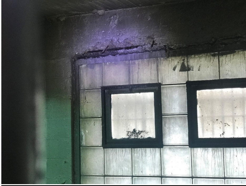
PHOTO # 5 – Damaged Lintel Closeup with Exposed Corroded Reinforcing Steel
