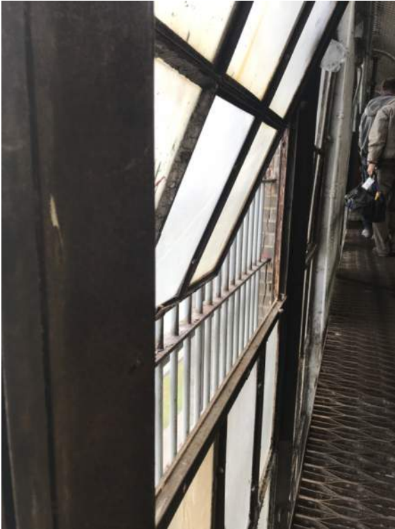
Photo 1-5e East Wall Window Condition
