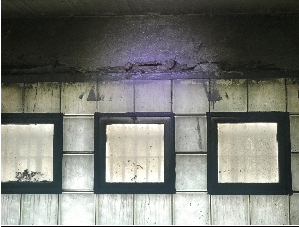
PHOTO # 3 – Damaged Lintel Closeup
