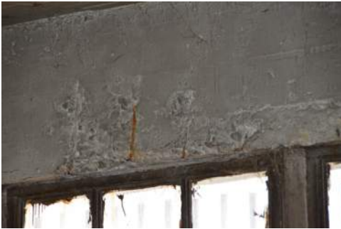
Photo 2-26: Interior D House West Lintels Require further investigation
