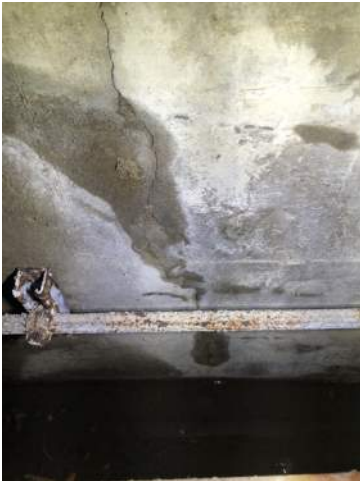
Photo 4-3b: Service Chase Foundation Wall Long Vertical Crack
