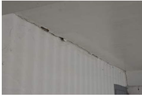
Photo 2-10: Interior D House Ceiling between Beams at Cell Wall crack
