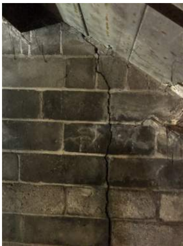
Photo 2-32: Interior Attic North Wall East side vertical crack
