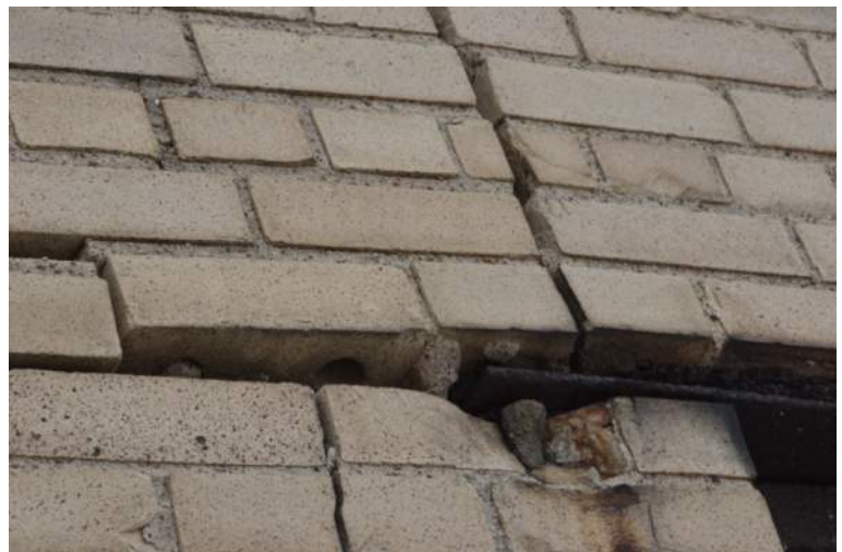
Photo 1-4d: Masonry Lintel with oxide jacking
