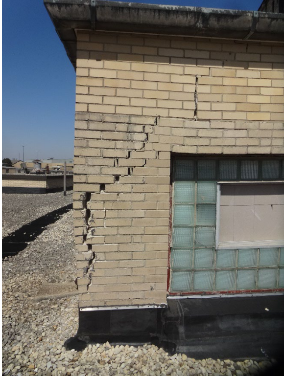
Typical location, displaced masonry.
