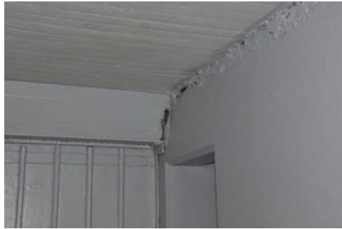
Photo 2-13: Interior E House Center Beam to North Wall from Cell Wall cracks
