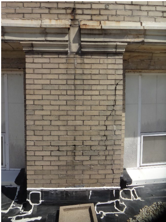
Typical location, cracked masonry.
