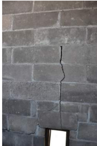
Photo 2-39: Interior South West Stairwell vertical crack at Lintel
