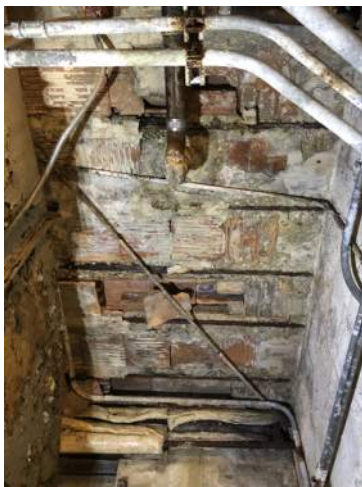
Photo 2-15: Interior B House Fan Room Ceiling/Shower Floors - Tiles broken
