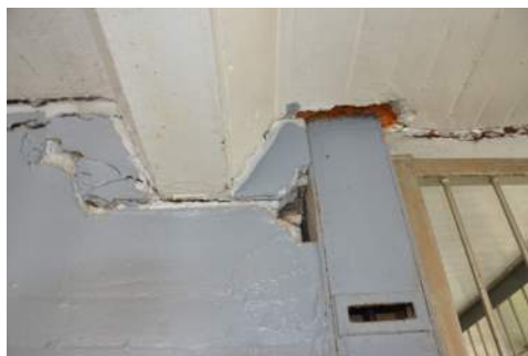
Photo 2-7: Interior C House East Beam to South Wall from Cell Wall cracks
