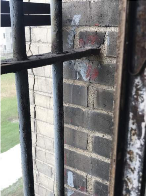
Photo 1-5a: Masonry Fine vertical cracks at Barred Grille
