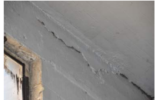
Photo 2-22: Interior Guard Rm cracks on exterior wall requires further investigation.
