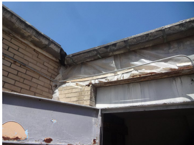
Typical damaged gutter and removed masonry.
