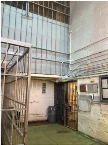
Photo 2-1a: Interior B House North Wall vertical crack
