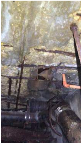
Photo 4-11: Service Chase Ceiling Slab Rusted & Partially Exposed Rebar
