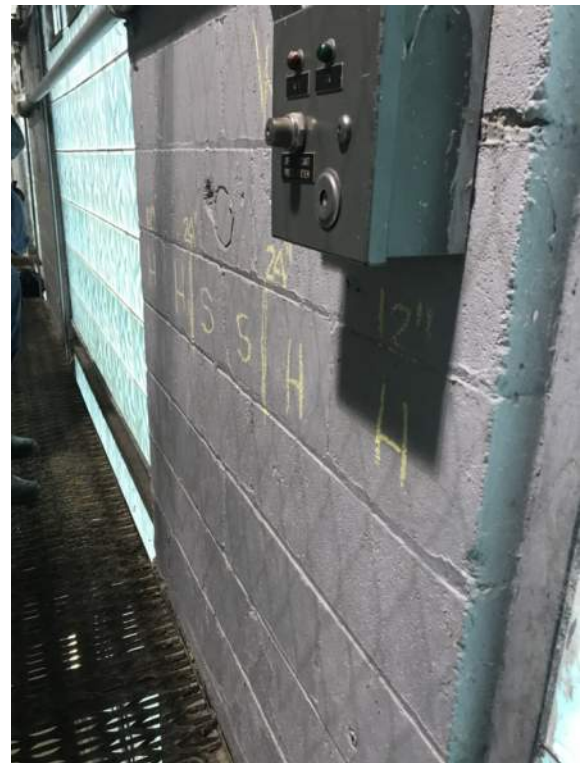
Photo 1-5h West Wall Glass Block Condition
