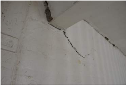
Photo 2-9: Interior D House West Beam to South Wall from Cell Wall cracks
