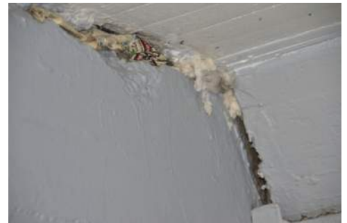
Photo 2-5: Interior B House Center Beam to North Wall from Cell Wall cracks
