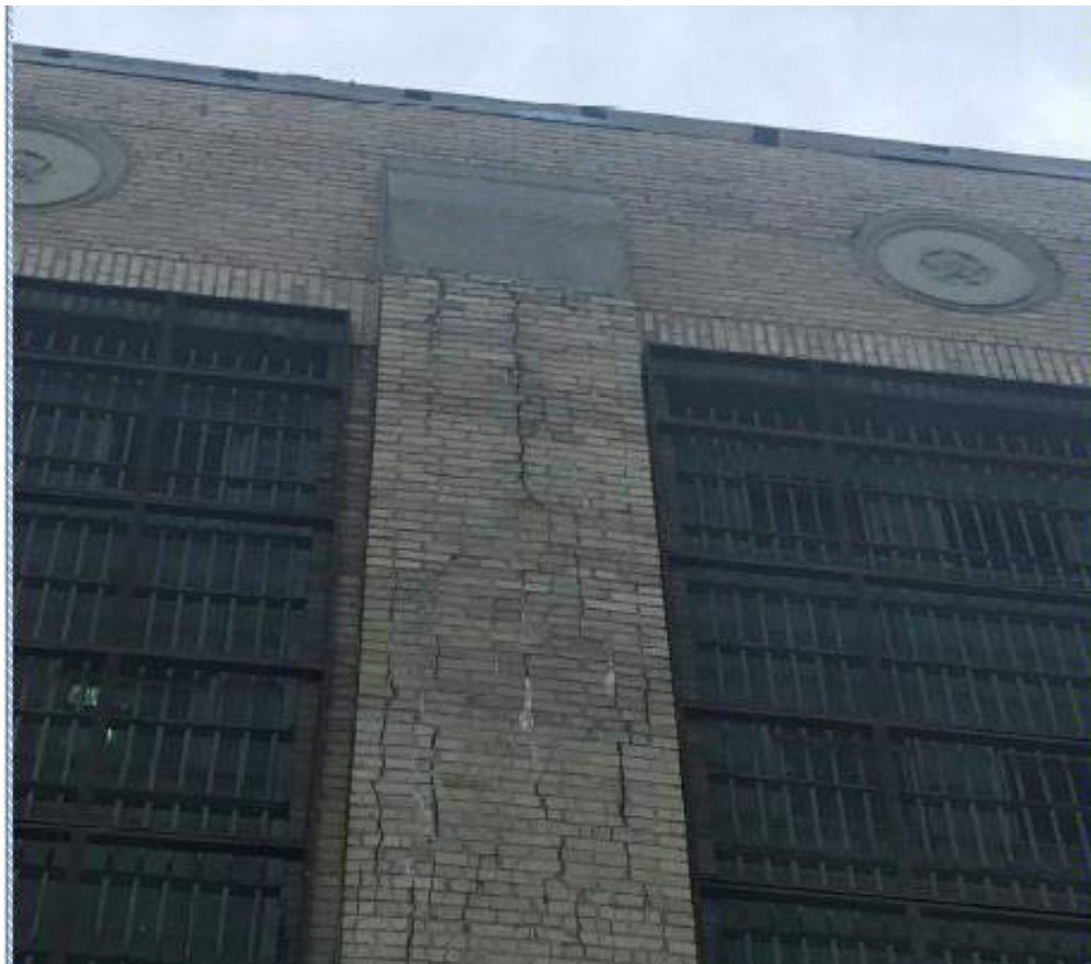
Fig. 2 Cracking distress noted in exterior brick face of pier.
