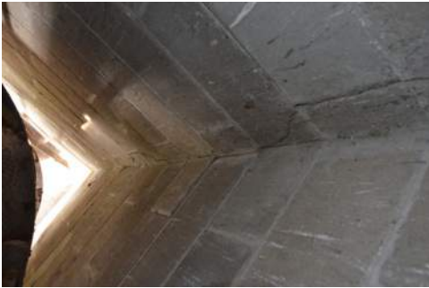
Photo 2-35: Interior South East Stairwell Corner vertical wall cracks
