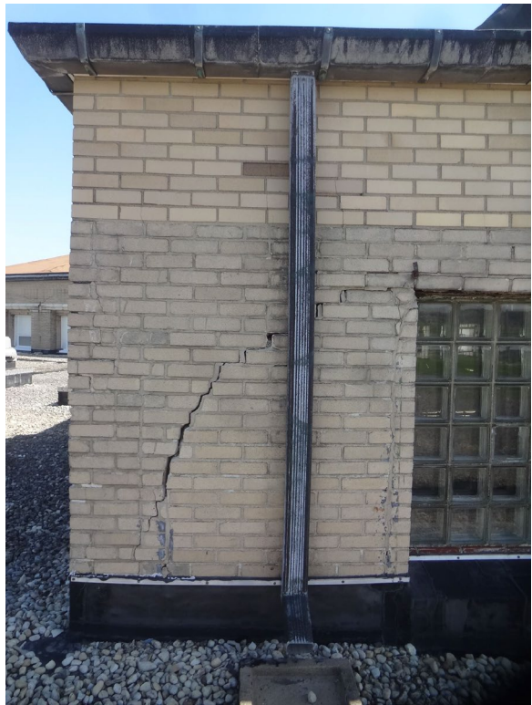
Typical location, displaced masonry.
