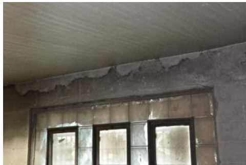
Photo 2-30: Interior E House West Lintels Require further investigation
