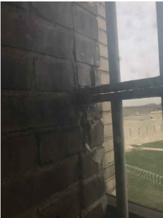
Photo 1-5c: Masonry Wide vertical crack at Barred Grille
