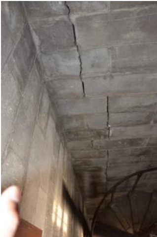
Photo 2-38: Interior South West Stairwell vertical wall crack
