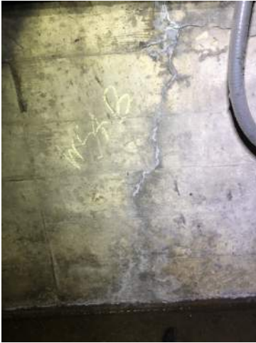
Photo 4-1: Service Chase Foundation Wall Crack Calcification
