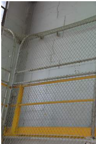
Photo 2-3: Interior C House South Wall vertical crack
