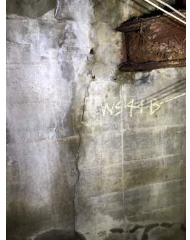
Photo 4-3a: Service Chase Foundation Wall Long Vertical Crack
