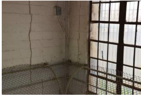
Photo 2-27: Interior D House South Wall vertical crack
