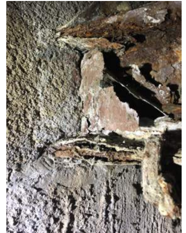
Photo 4-13: Service Chase Beam Fixed End Bearing Oxide Jacking
