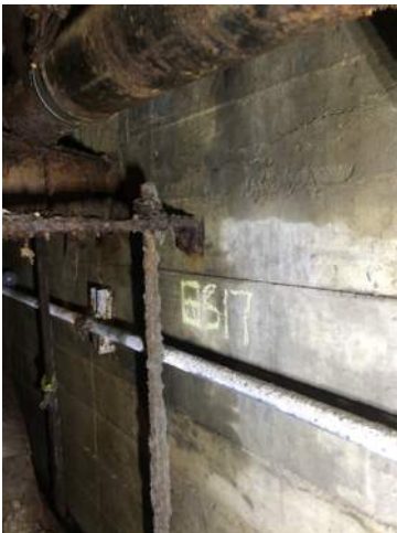
Photo 4-5: Service Chase Foundation Wall Horizontal Crack
