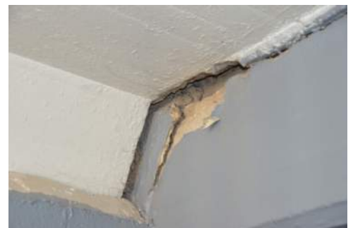
Photo 2-8: Interior C House Center Beam to South Wall from Cell Wall cracks
