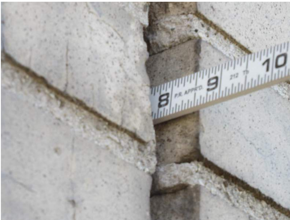
Fig. 9 Pier W7 front face vertical crack exhibiting out-of-plane offset.
