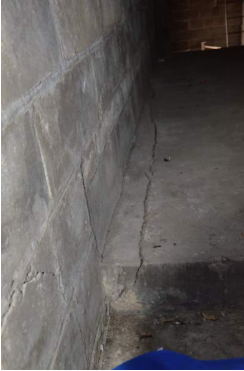
Photo 1-3f: Masonry South Arch Interior Slab crack
