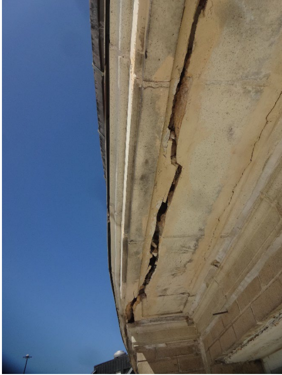
Typical location, damaged terra cotta.
