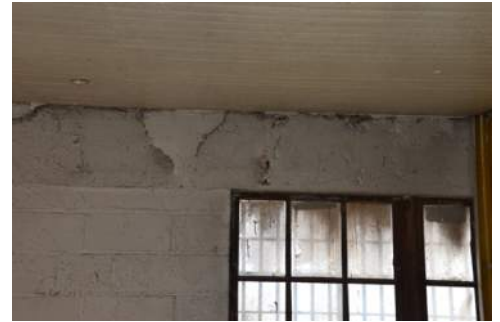
Photo 2-28: Interior D House West Lintels Require further investigation
