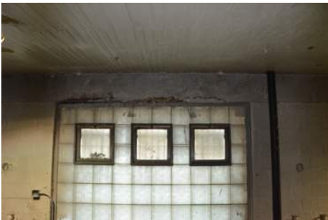
Photo 2-29: Interior E House West Lintels Require further investigation
