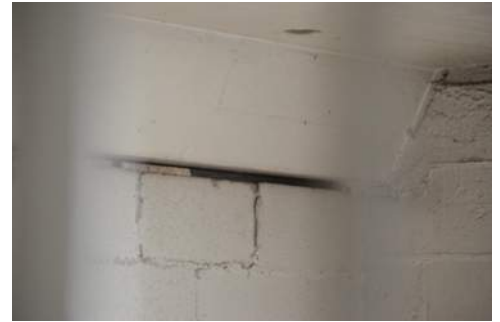
Photo 2-11: Interior D House Center Beam to South Wall from Cell Wall cracks
