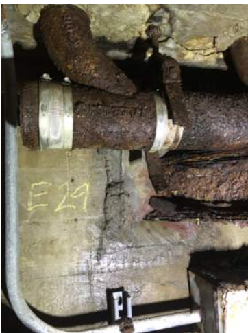
Photo 4-14: Service Chase Beam Fixed End Bearing Oxide Jacking
