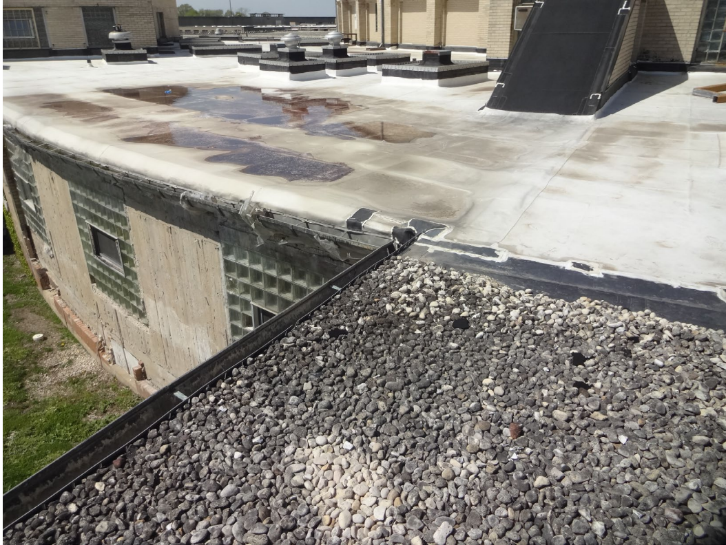
Typical area of temporary roofing repair.
