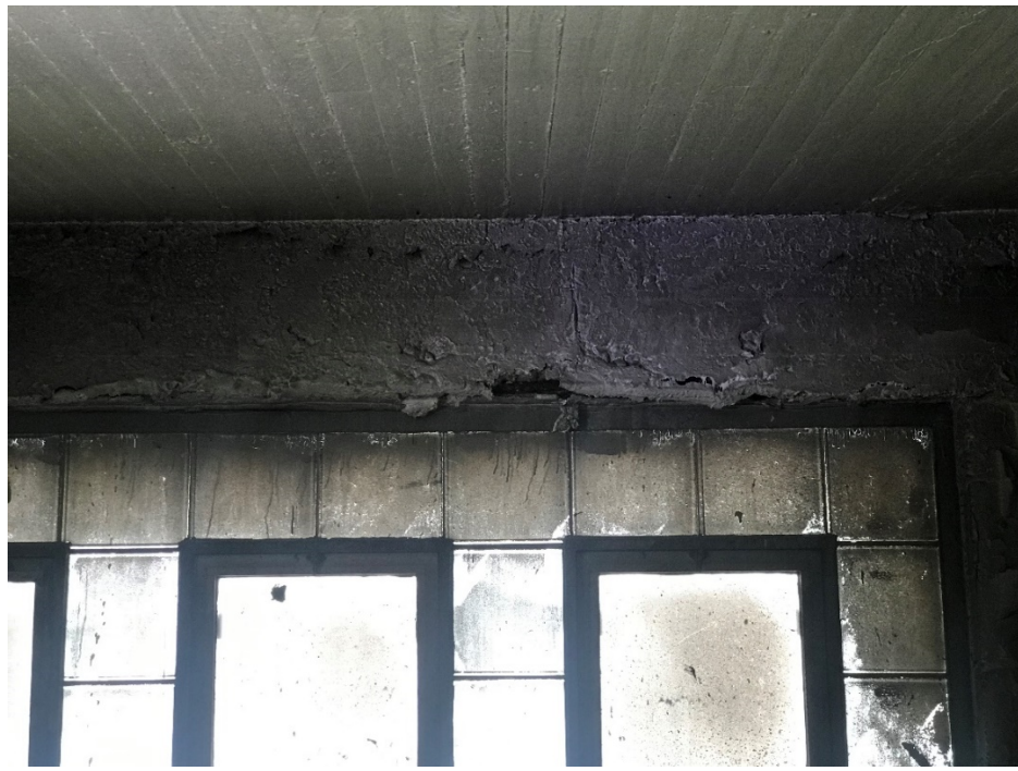
PHOTO # 6 – Damaged Lintel Closeup
